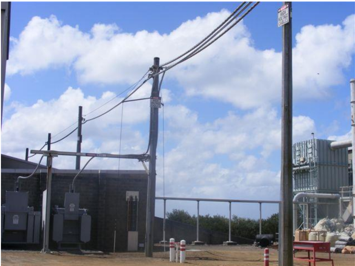
PORTLAND 22kV AERIAL LINES SHOWING THE INSULATED CABLE CONSTRUCTION AND LACK OF SIGNIFICANT VEGETATION
