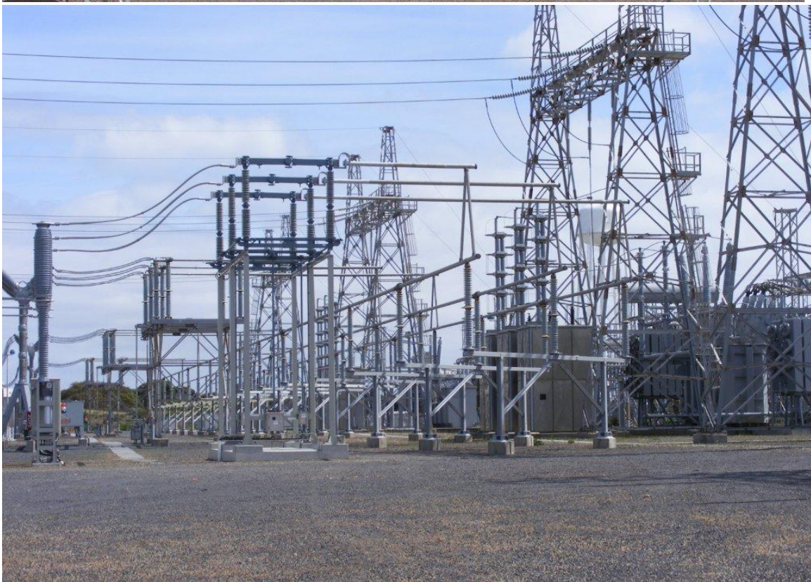
PORTLAND MAIN SWITCHYARD ILLUSTRATING LACK OF SIGNIFICANT VEGETATION
