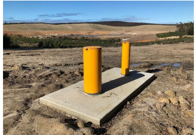
A pair of monitoring bores.
